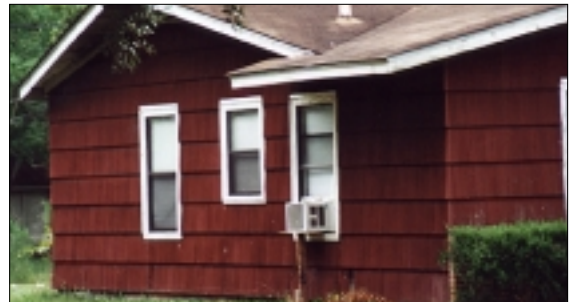
Covering over the original exterior of a home will damage its historic integrity.
