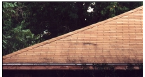
Neglecting roof repairs can become costly and detracts from the appearance of a residence.
