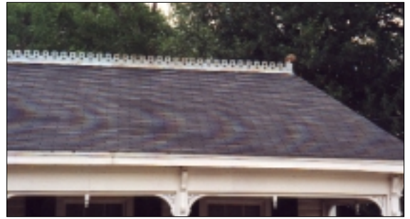
The original roof reflects the historic character of a residence and should always be well maintained.
