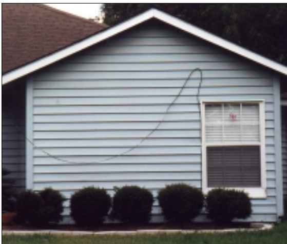
In this case, the use of synthetic siding resulted in the loss of original components of the residence.
