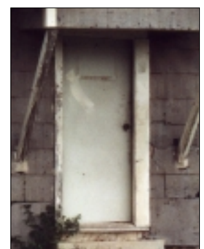
Do not allowing doors to fall into disrepair.
