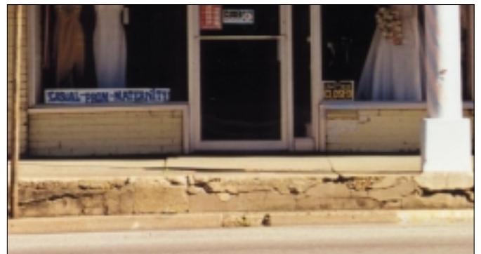
Kickplates should never be removed or covered over with brick or other material.
