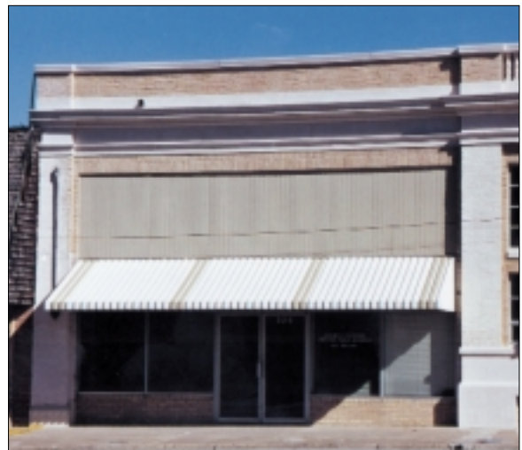
When transom windows are covered or painted over, the building loses historic integrity and the appearance of the entire streetscape suffers.
