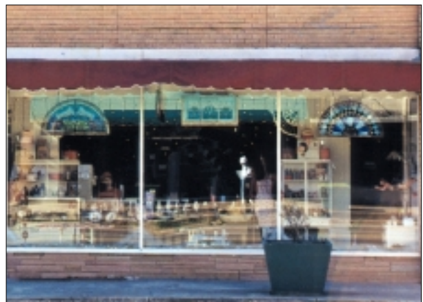
Inappropriate alterations to display windows include modification of the original size and replacement with aluminum framed windows.
