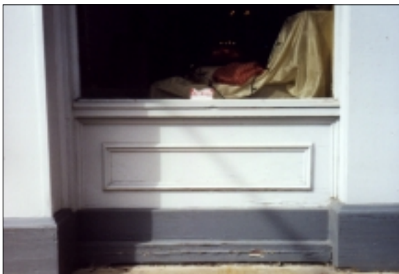
Kickplates supply a sense of balance and create visual interest on a storefront.
