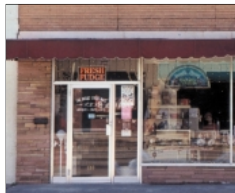
Entryways should never be modified with aluminum doors.
